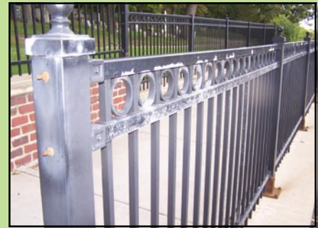
PREVENT Failed Coatings with Proper Procedures
